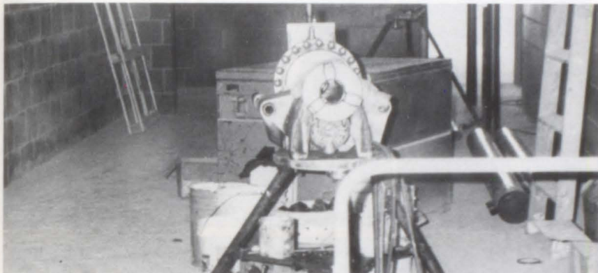
Getting ready to be moved into, the new school is going up!
